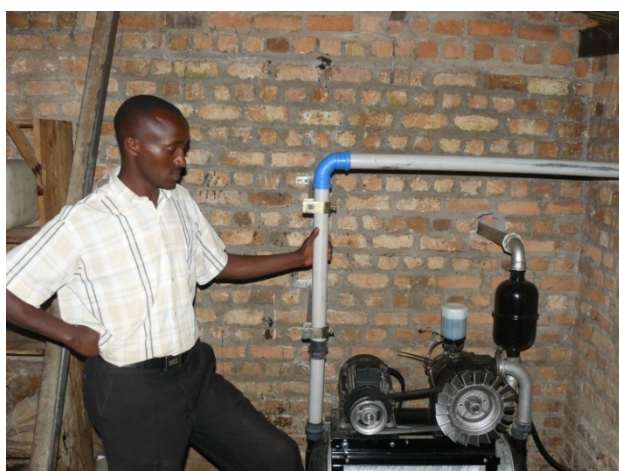
Fig. Milking Machine installed in Bukeye
