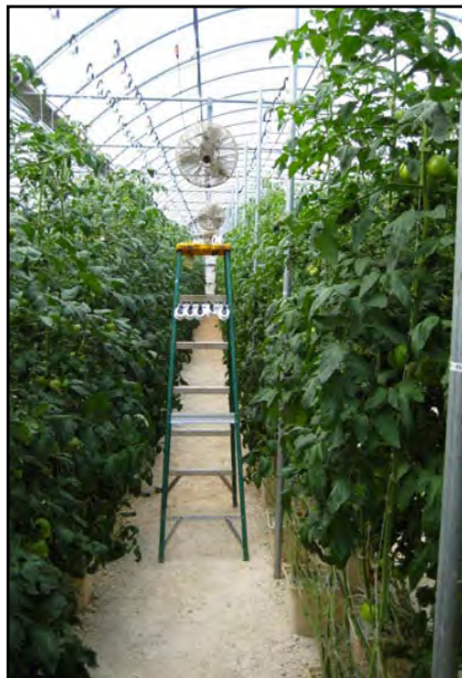
Horizontal air flow fans provide air movement within the structure.
