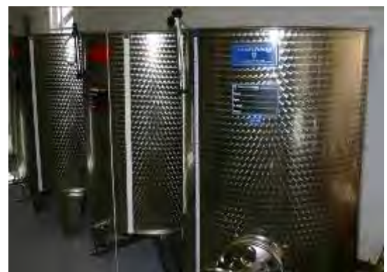
Stainless steel storage tanks for oil
