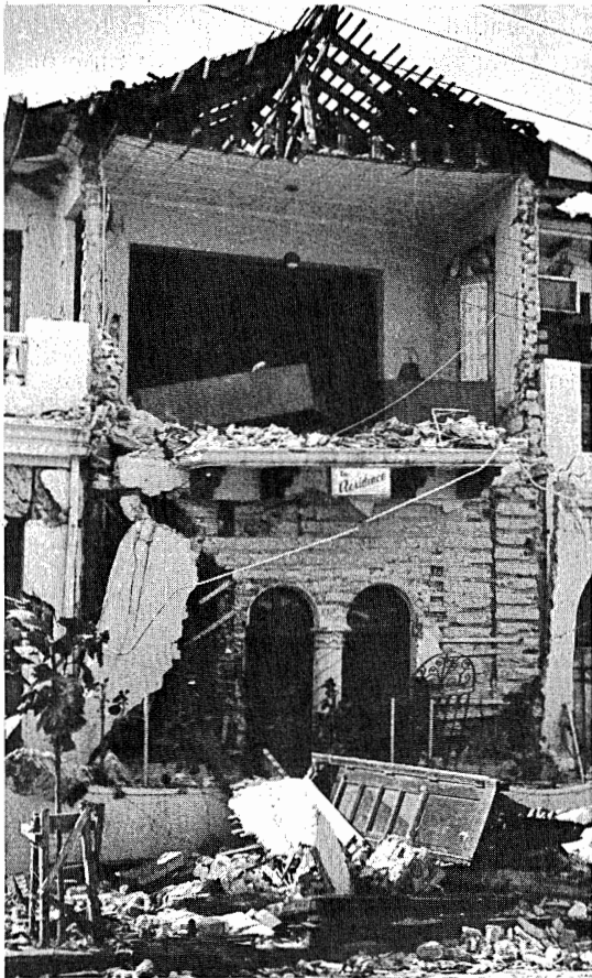
The weakness of the once popular block and lathe construction was easily discernible.
