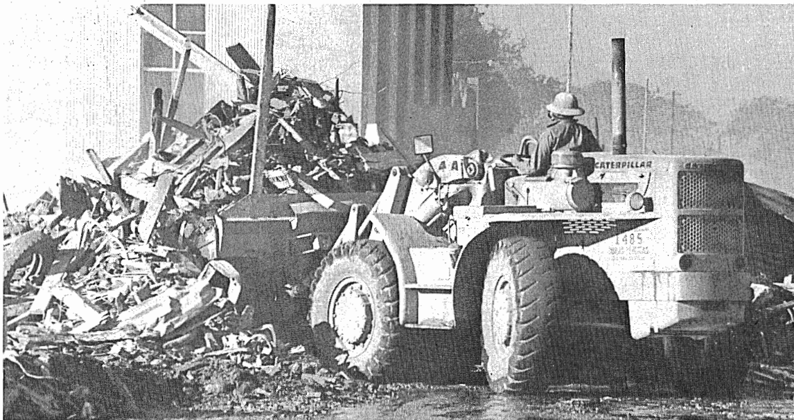
Mobile heavy construction equipment was used to clear rubble and debris off the streets.
