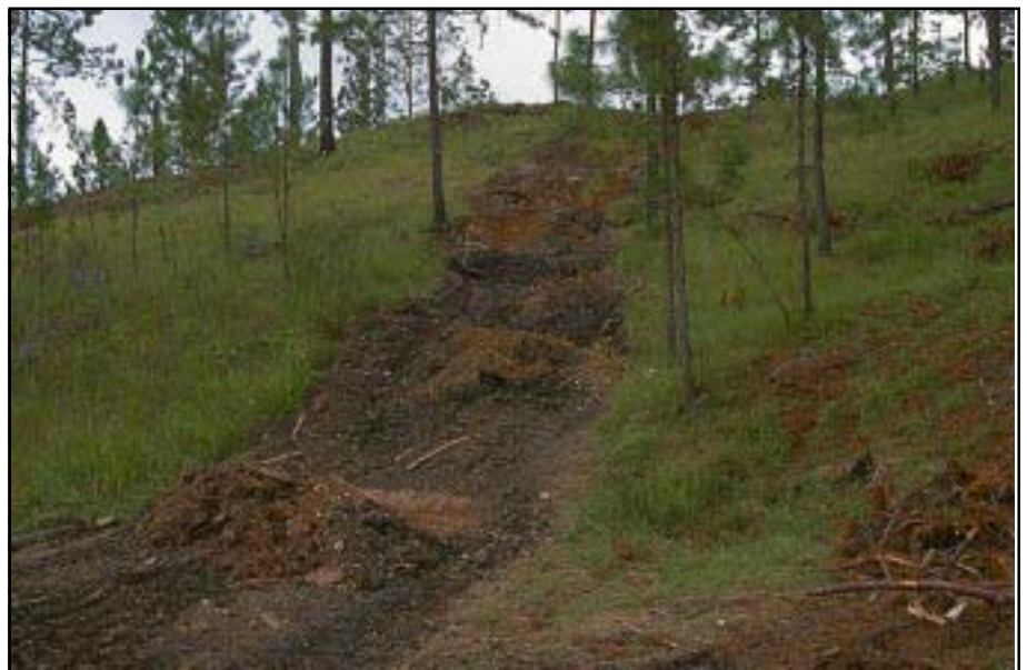
Photo 3.8 Stabilize skid roads and trails after use with water bars and apply a ground cover or other erosion control measures.
