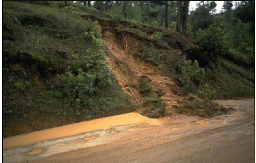
Photo 4.11 Remove slide material that blocks the drainage ditches and narrows the road.
