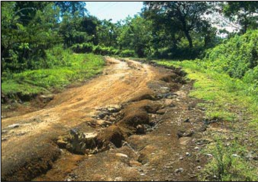
Photo 1.2 A poorly drained road that has a rough driving surface for the users, it is a source of sediment, and it is relatively expensive to maintain.
