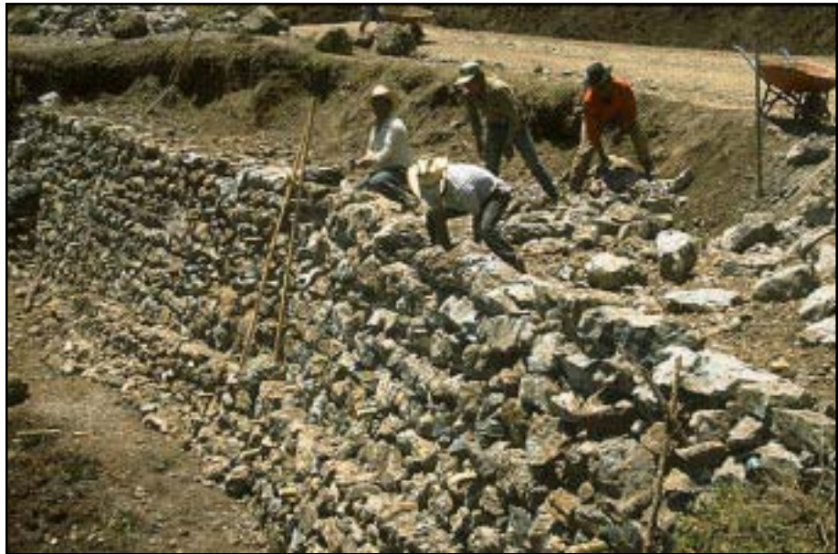
Photo 11.8 Use physical slope stabilization methods, such as retaining walls, reinforced fills, or rock buttresses where necessary in areas of space limitation on steep slopes.
