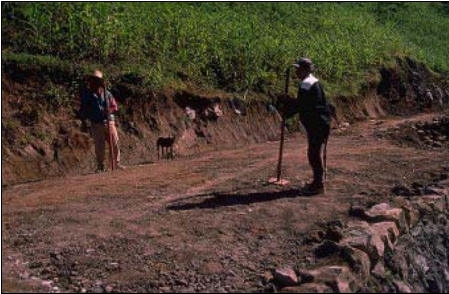
Photo 11.6 Simple hand compaction behind a low rock wall. Compaction is important behind any retaining structure or fill. It can be achieved by hand or, preferably, using equipment such as a wacker or small compactor.
