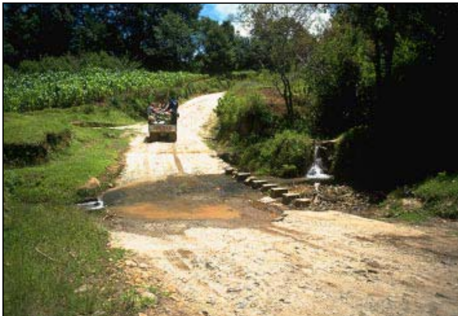
Photo 9.1 Use armored low-water crossings, fords, or drifts as often as possible to cross low flows in broad, shallow natural drainages, thus avoiding the use of pipes. Note that part of this reinforced driving surface needs repair.
