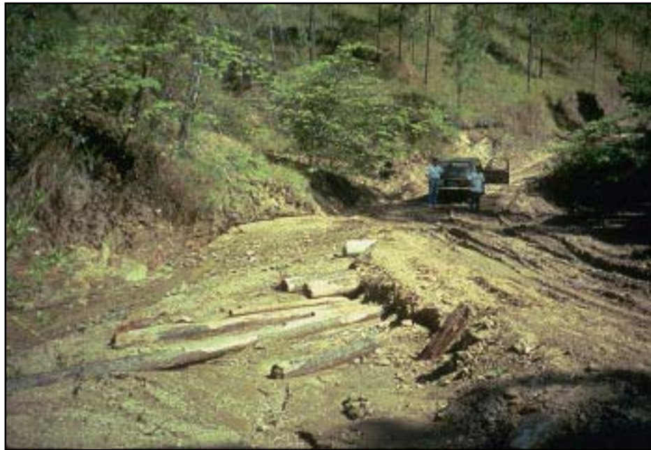
Photo 8.10 Most log culverts have very little flow capacity. Remove temporary log (Humboldt) culverts before major rainstorms or before the rainy season.
