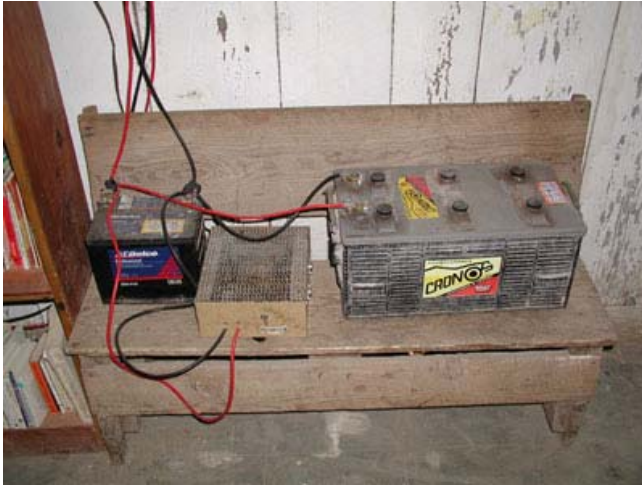
Fig. 3: A collection of power system components on a bench at one side of a Telesecundaria classroom in Durango. The box in the middle is actually a homemade inverter.
