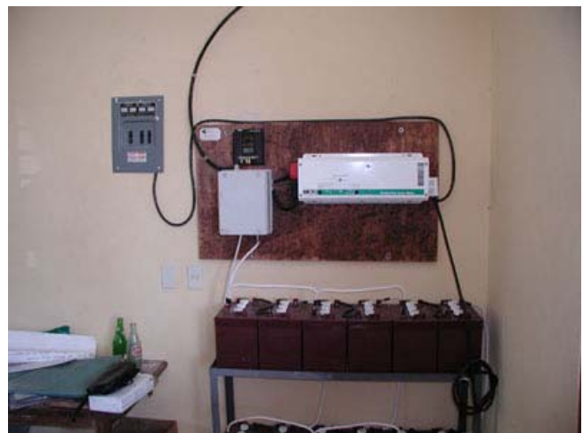
Fig. 4: A well-organized layout of power system components in a newly installed PV-powered Telesecundaria in Quintana Roo.
