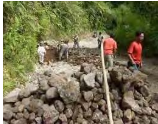
Farm road hardening construction in Tj. Barus Villages, one of the central production villages for citrus in Karo District
