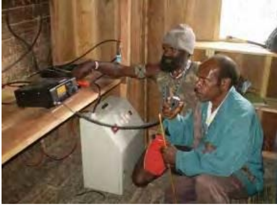
Radio communication installed at Pireme
