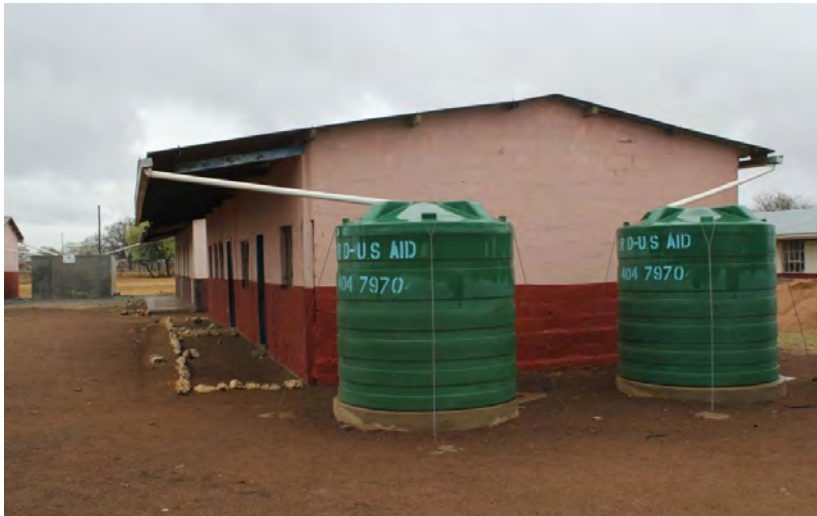
Picture 19. Ngcina Primary School is one of the many schools, which benefited from IRD's intervention in the provision of potable water through the installation of rain water harvesting system
