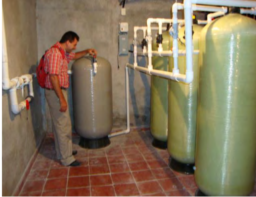
Installed water purification system - El Tablón. Photo credit: Adel Chalatenango
