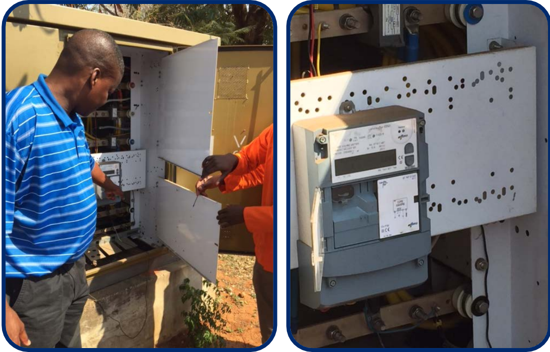
Figure 26 AMR Meter installed
