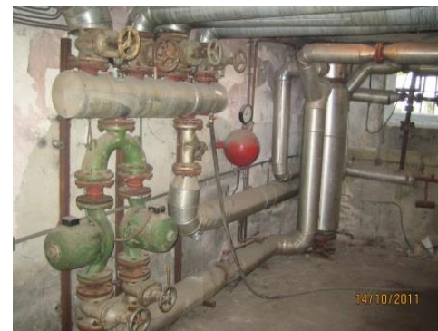
Old heating substation
