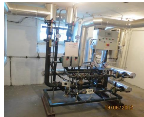
New heating substation
