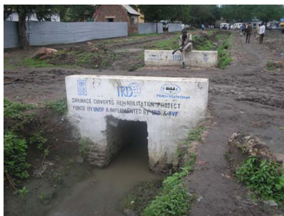
ABOVE: IRD said that they tried to coordinate with county, who was going to dig a master and drain that all these types of drains feed into. However, they did not do it.
