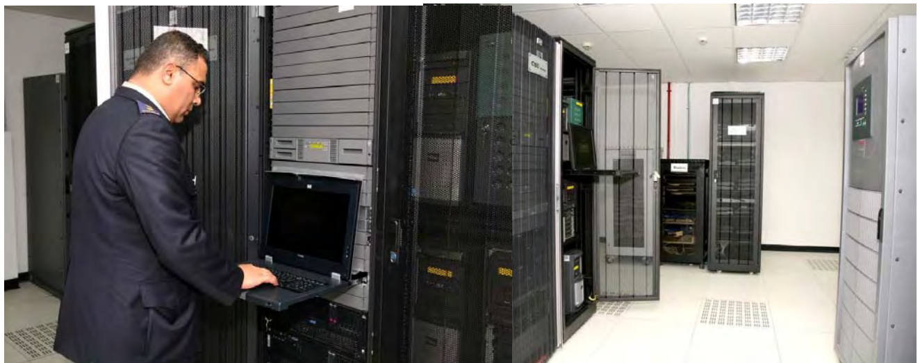
The new, fully modernized, state-of-the-art data center at Jordan Customs.
