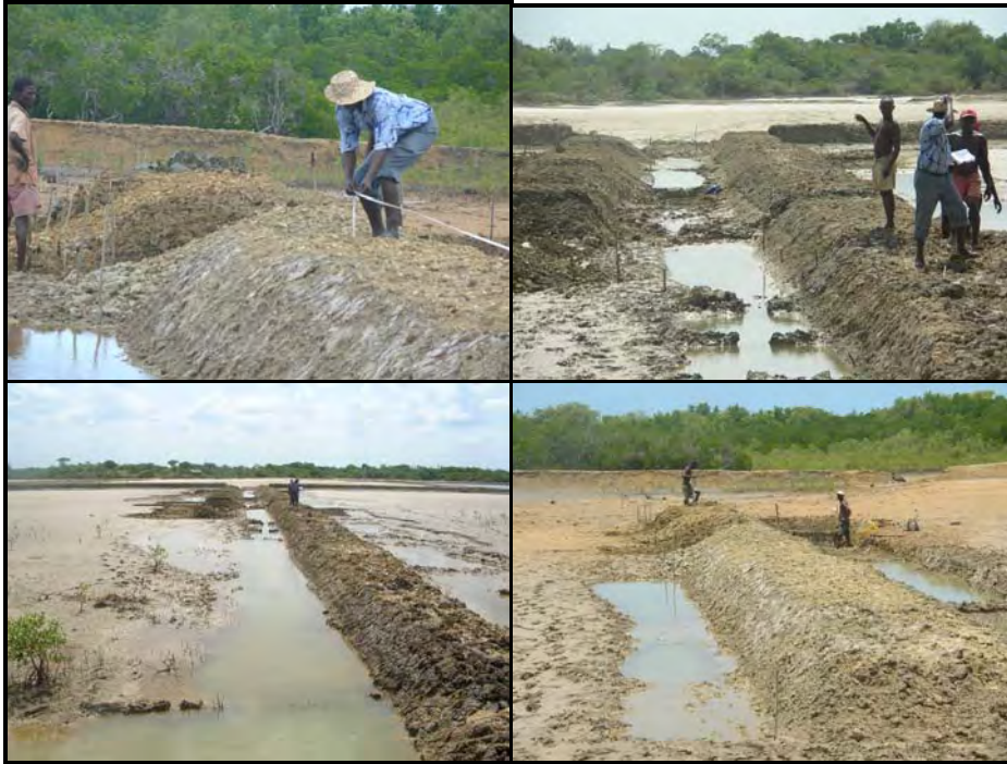
Figure 20: Main canal and dike with the main gate in the foreground in April 2006 at the farm of Mr Mkadam, Mkuranga, Tanzania.
