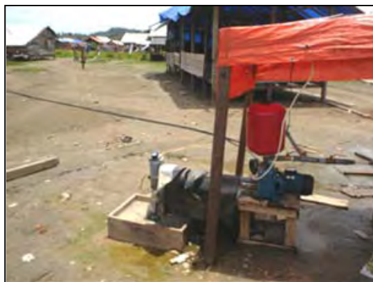
Figure 5: Well and Pump System at Lhok Buya near Calang.
