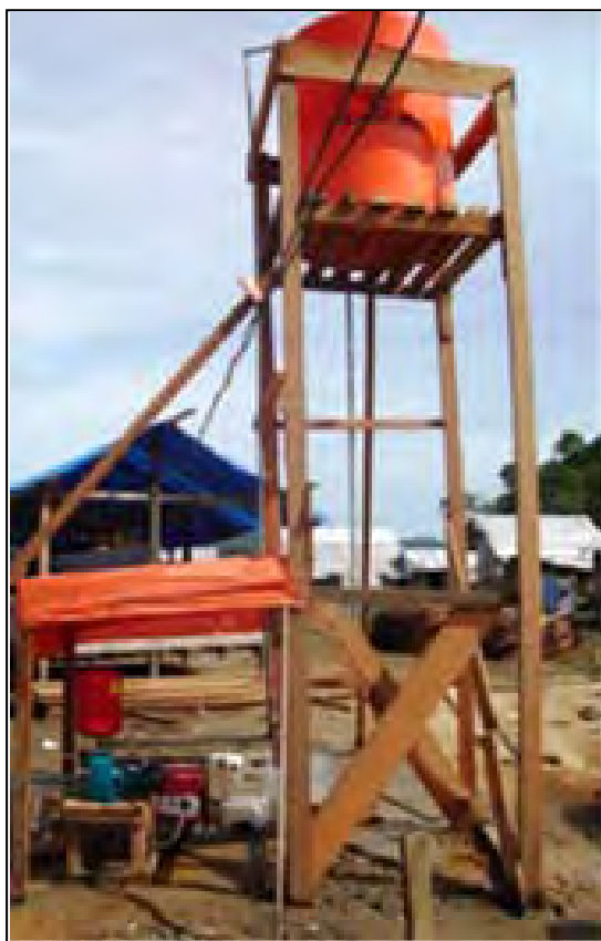
Figure 6: Final Water Supply System at Lhok Buya (IRC photo).
