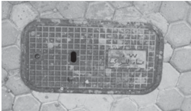
Reclaimed water valve access box on sidewalk on Embassy Row in Riyadh, Saudi Arabia. Photo courtesy of Bahman Sheikh
