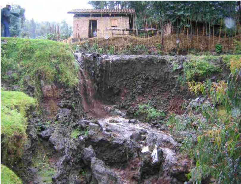
Figure 1: Severe erosion of volcanic soils in Rwanda. The steep pouroff is a headcut migrating up stream and across a road.
