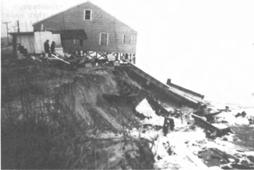
FIGURE 2-4 Structures built on sea cliffs may be subject to hurricane winds and the resulting erosion. Improved weather prediction capabilities are available, but good communications systems and emergency preparedness plans are also needed so that early warning systems can allow coastal inhabitants to evacuate danger zones in time. (U.S. National Oceanic and Atmospheric Administration)
