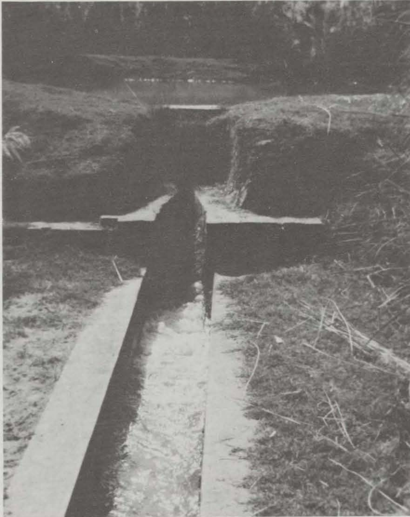
Water from distributary canal flows through mogha into lined section of an improved watercourse.
