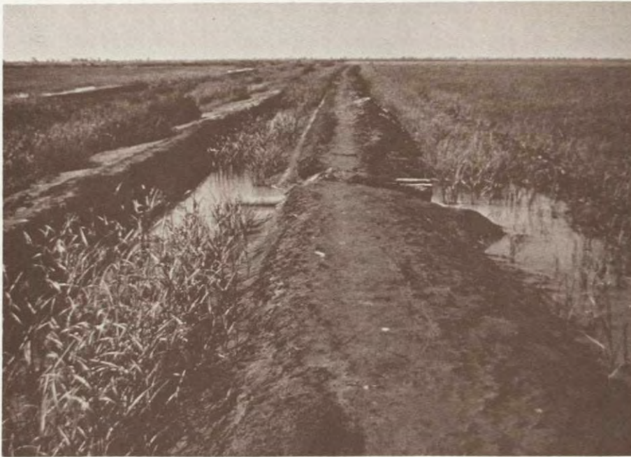
Improperly maintained irrigation canals clogged with the semi-aquatic plant, Cyperus.
