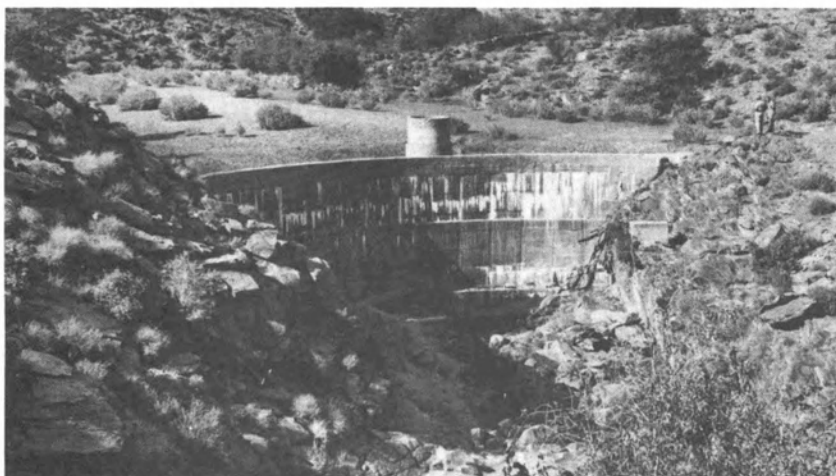
FIGURE 44 Sand-filled storage dam in South-West Africa built of concrete. Staged construction is clearly visible. Well shaft behind the dam wall is used to extract the water. The dam size can be judged from the persons at right. (O. Wipplinger)
