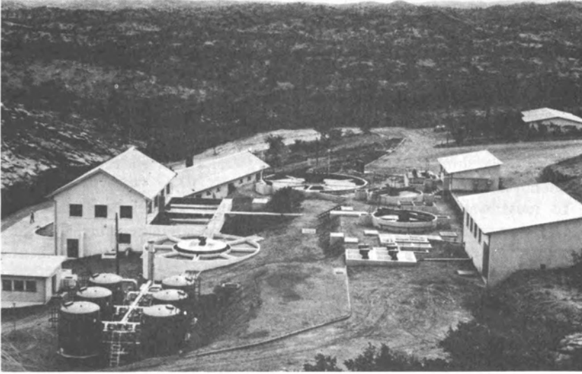
FIGURE 32 City of Windhoek, South-West Africa, (population 84,000) on the edge of the Namib Desert cycles its municipal wastewater through this treatment plant and back into the potable supply. (National Institute for Water Research, Pretoria, South Africa)
