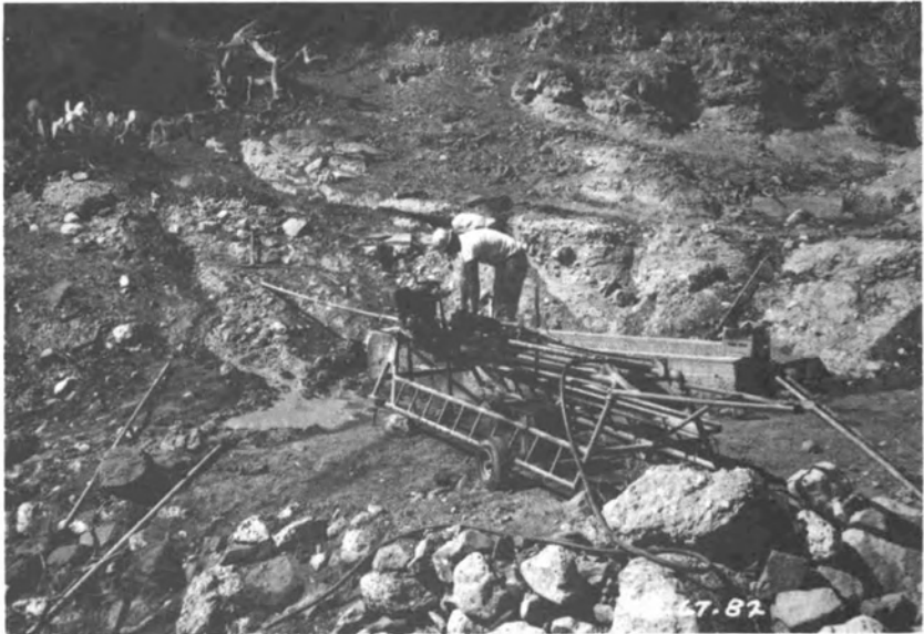
FIGURE 38 Drilling a horizontal well. A standard well casing is drilled on a slight downward slope. Equipment is light and portable and easily transported even in remote, rough terrain. (W. T. Welchert)
