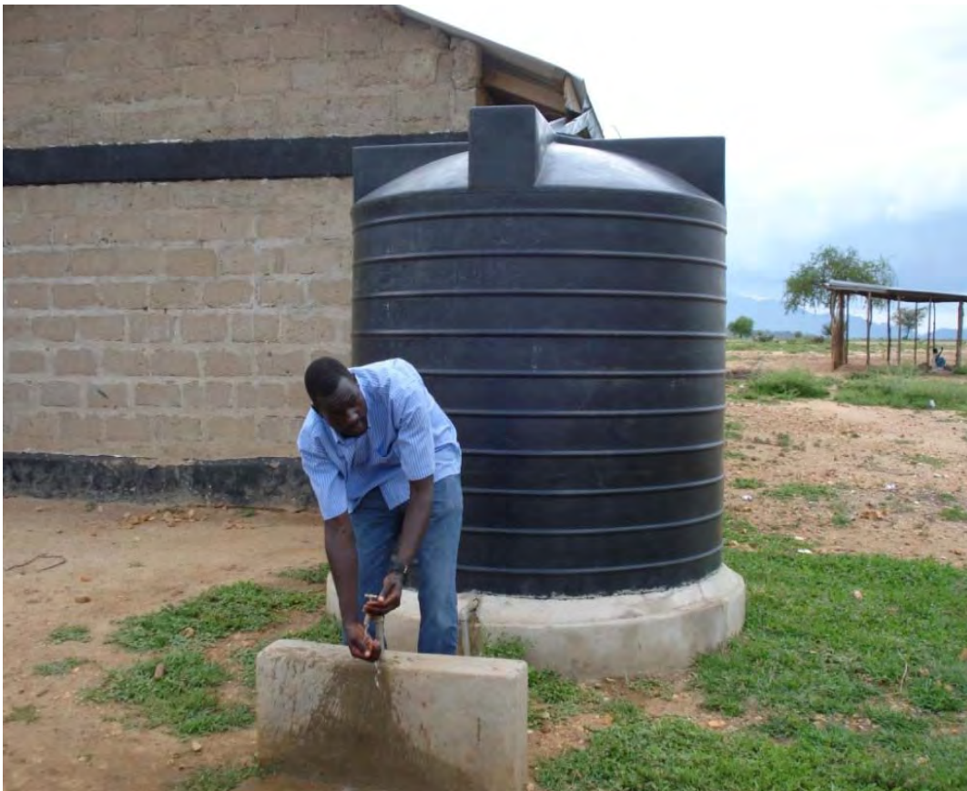
Roof catchment tank, Namorunyang school, Kapoeta South, built by LRDA.
