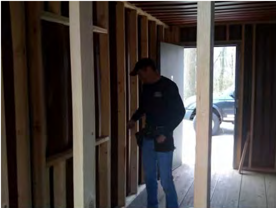
A Carpenter frames the walls in a container that will become one of the three studios of SRS FM Juba.
