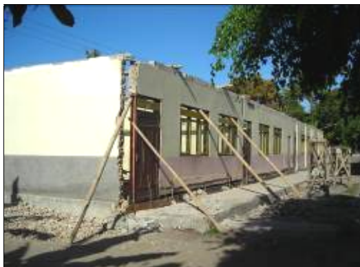
SDN 01 Granting, Klaten, before the rehabilitation process, May 2008
