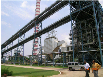
Bagasse handling unit at Godavri Sugar's 24 MW bagasse cogeneration plant in Karnataka, Photo: Sandeep Tandon
