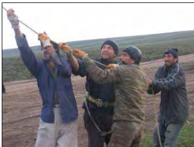
Workers raise a utility pole for a Jalilabad flour mill's new electric line, southern Azerbaijan
