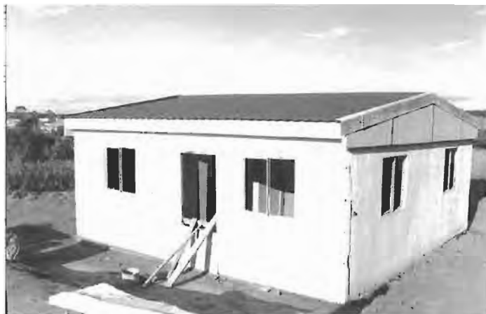
Almost completed “show” home – touch up external plaster, glazing and front door to be installed. This will be done when beneficiary is found or when used as site office for Amalinda infrastructure installation.
