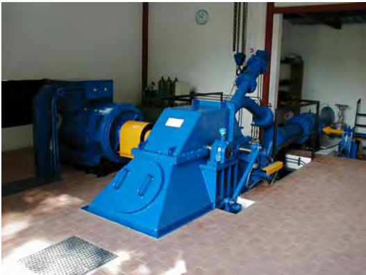
E+Co funded, 485 kW, La Nieve Hydroelectric plant, Honduras
