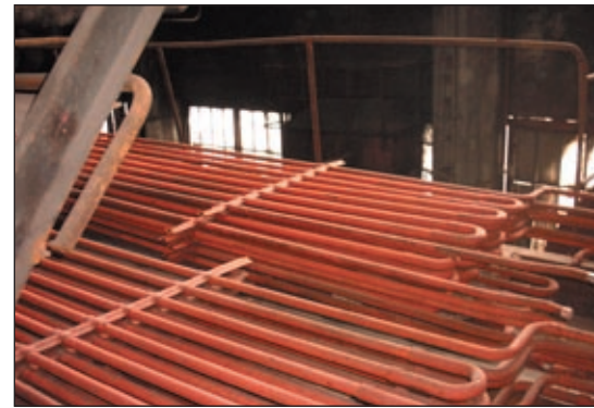
United Bank of Bulgaria’s guarantee has catalyzed lending to commercially viable enterprises and service companies for municipal infrastructure improvements such as this heat exchanger in Goma Orjahovitza.
