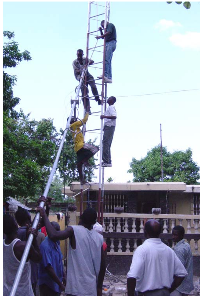
RAMAK personnel worked hand-in-hand with the organizers of Radio SAKA in Grand Goave to install a new tower that doubled their broadcast range.
