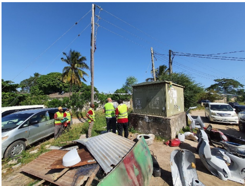
Zanzibar Electricity Corporation employees verify two low-voltage lines connected to a distribution transformer in Makadara. Photo credit: EAEP
