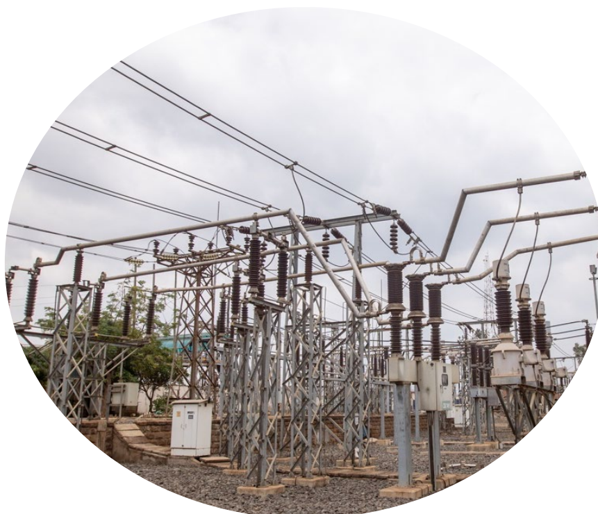
Power infrastructure at Roysambu substation in Nairobi, Kenya. Photo credit: EAEP
