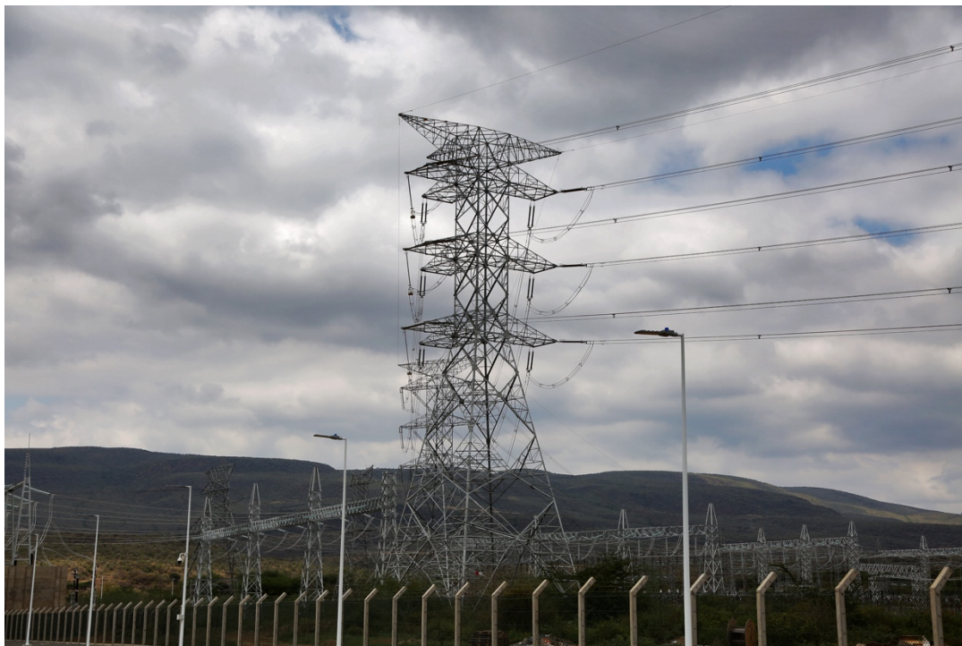
Power transmission lines cutting across the land, Suswa Kenya. Photo credit: Nyaga Ireri
