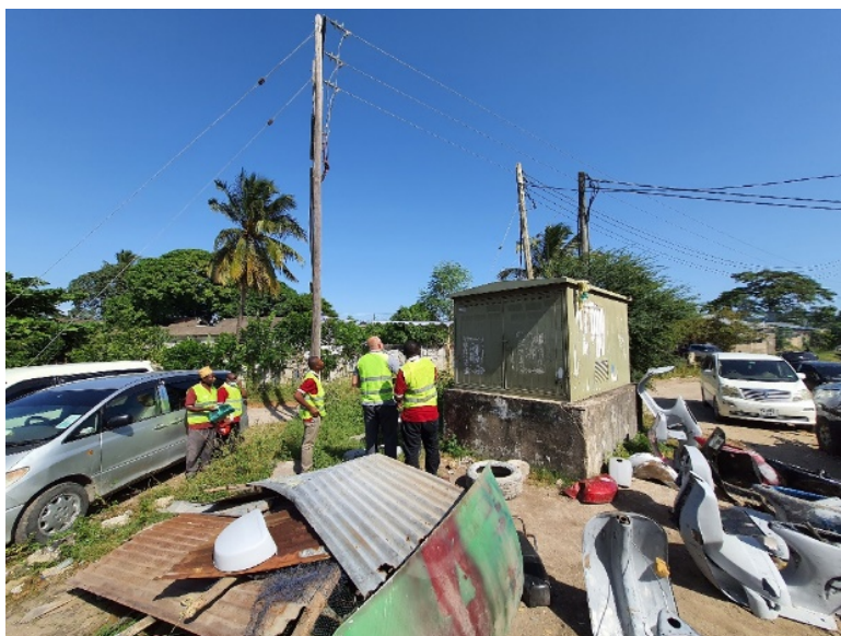
Zanzibar Electricity Corporation employees verify two low-voltage lines connected to a distribution transformer in Makadara. Photo credit: EAEP
