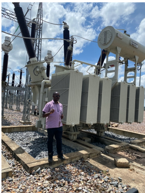
EAEP team inspecting the Mbarara sub-station under Shango-Mbarara interconnection commissioning activity. Photo credit EAEP
