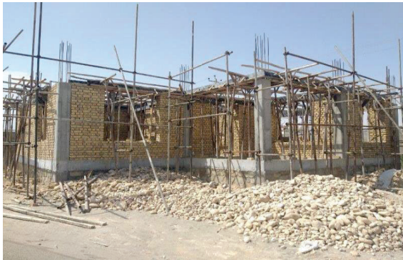
Photo #5: First floor slab formwork of the office building, Mazar-e-Sharif, Balkh Province. ZA, 2021-05-22.
