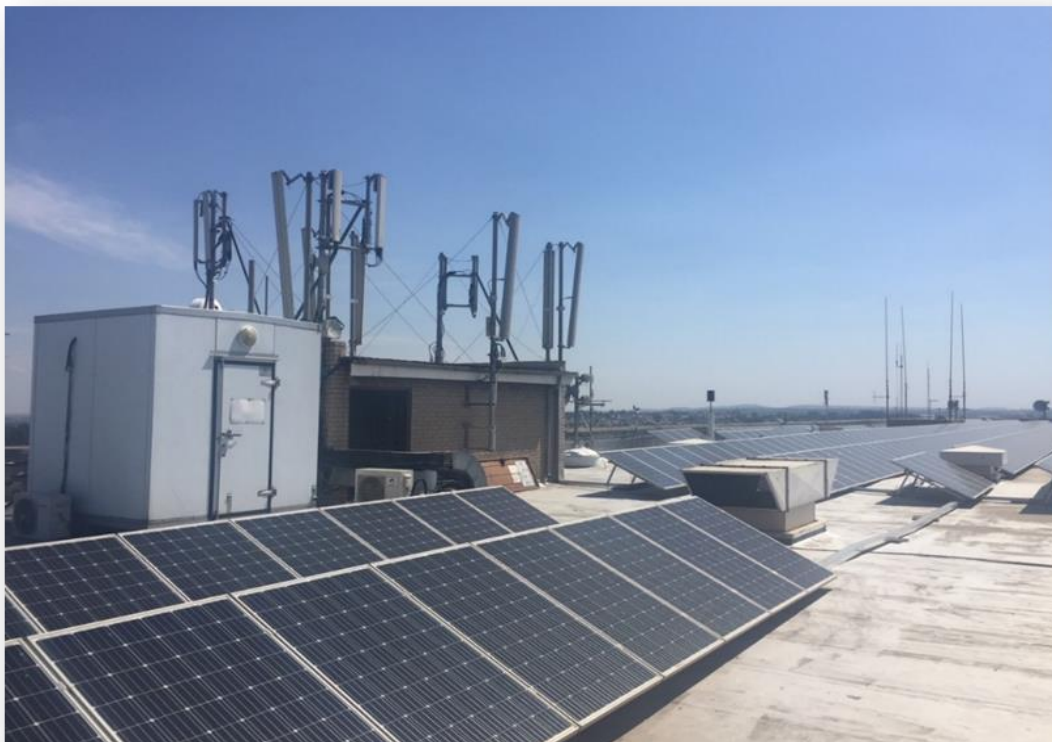
Photo 1: An example of a solar PV installation at Ekurhuleni Metropolitan Municipality office.
