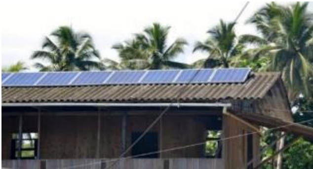
Figure 18 Cajambre PV system and refrigeration installations
