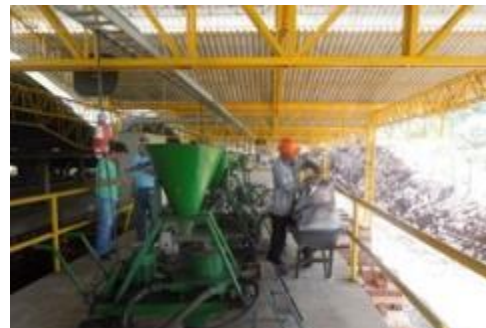
Figure 20 Automated pulverized coal injection system at Sugres
