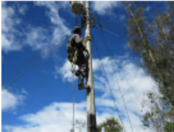
Colombia Clean Energy Program
