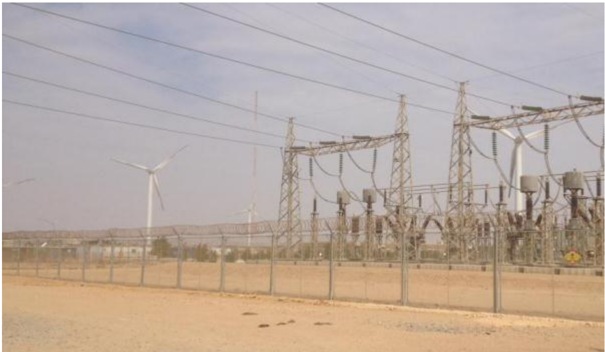
Fauji Fertilizer Company Energy Limited (FFCEL) HV Switchyard at Jhimpir
