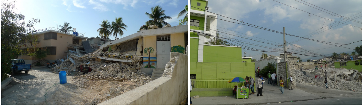
Figure 1a (left). Collapsed private school in central Port-au-Prince metropolitan region; a neighboring single-family house sustained no damage; (b, right) Well-built commercial building (left side) adjacent to catastrophic collapse of neighboring structure.
