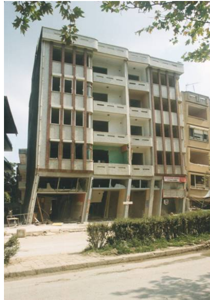
Figure 13. A Reinforced Concrete Frame Building at Near Collapse
