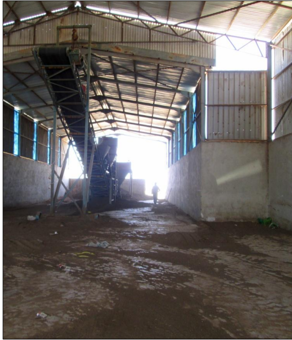
Figure 3-7: Mechanical processing equipment
