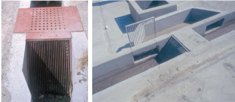
Figure 28.h. Typical Bar Screen Installations
