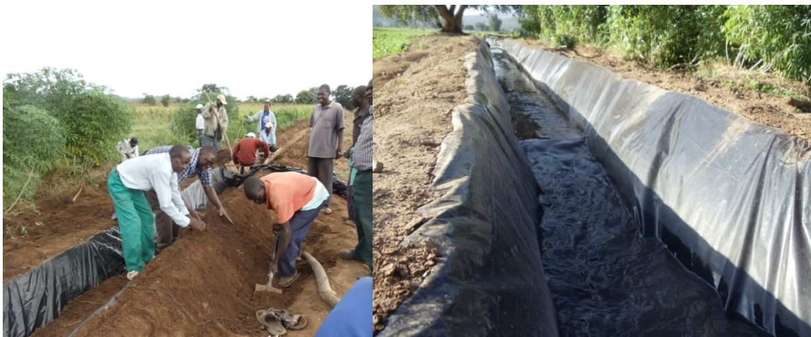
Left: Bwerudza farmers lining one of the earth canals with UV-protected plastic sheeting to reduce conveyance water losses; Right: the finished conveyance plastic-lined canal with water flowing through it.
