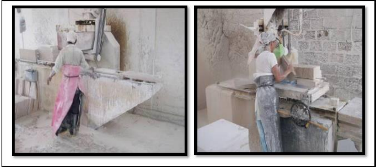
Figure 24 Poor Working Environment at the Processing Plant
