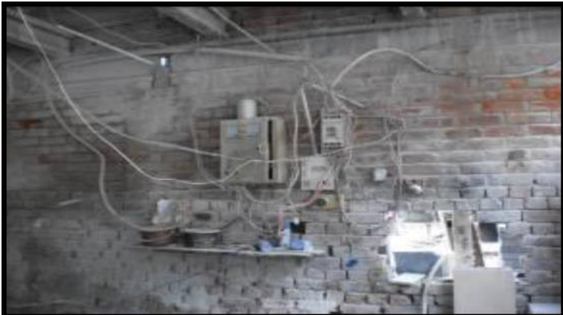
Figure 25 Safety Hazard at a Processing Plant
