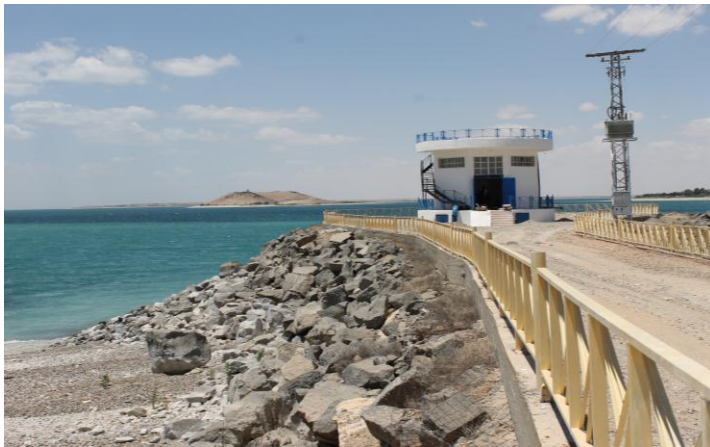
Jabaar Pump Station after the repairs conducted by ES-North. The site now has operational water pumps to deliver irrigation water to the surrounding communities. ES-North also upgraded the safety features at the site.
