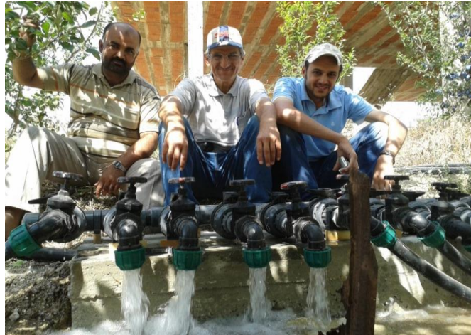
Water flowing from the solar powered water pumps procured and installed by ES-North.
