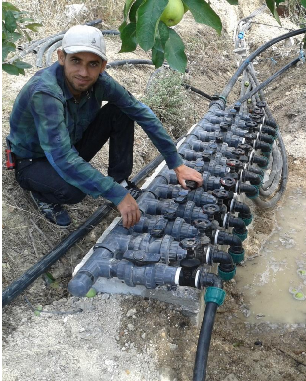
ES-North embedded staff works on the installation of pipe manifolds for irrigation equipment in Idlib province
