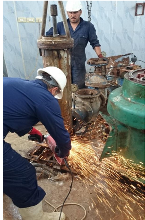
Workers repair a water pump in the Jabaar Pumping Station on Lake Assad.
