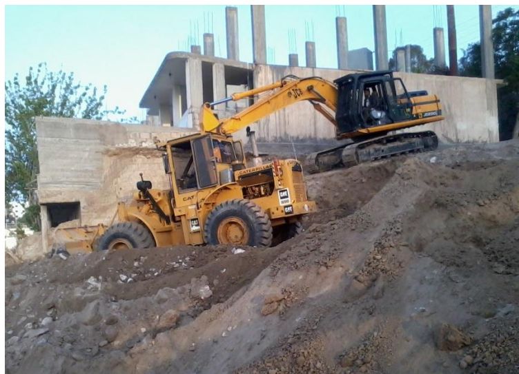
Heavy machinery is used to prepare the rehabilitation site in Al Mayadin.
