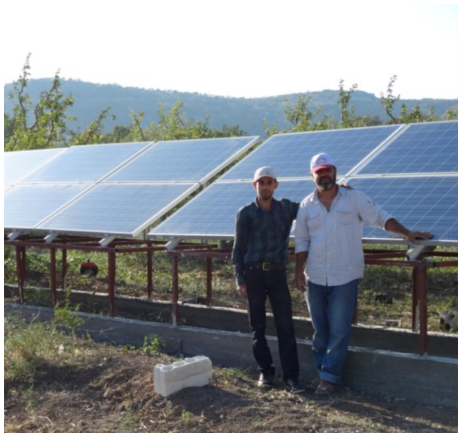
ES-North staff stand next to completed solar panels for the Bdama orchard irrigation system.
