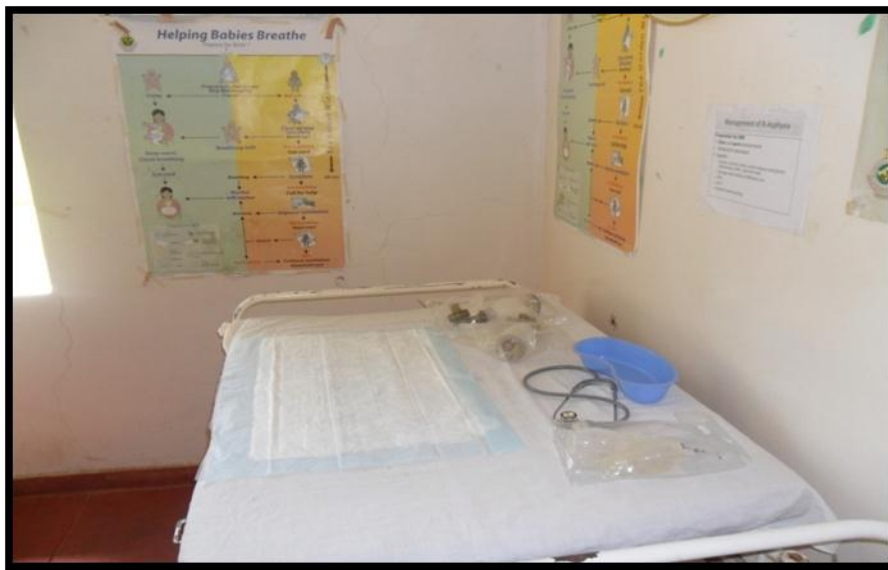
Rusitu Mission Hospital Newborn Care Corner: Space and equipment ready for newborn resuscitation.
