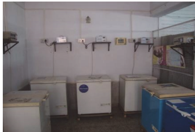
Picture 13: Cold chain room after intervention
