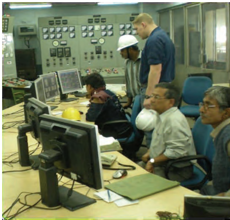
U.S. expert monitoring the combustion process at Control Room, Kolaghat, West Bengal under APP.
