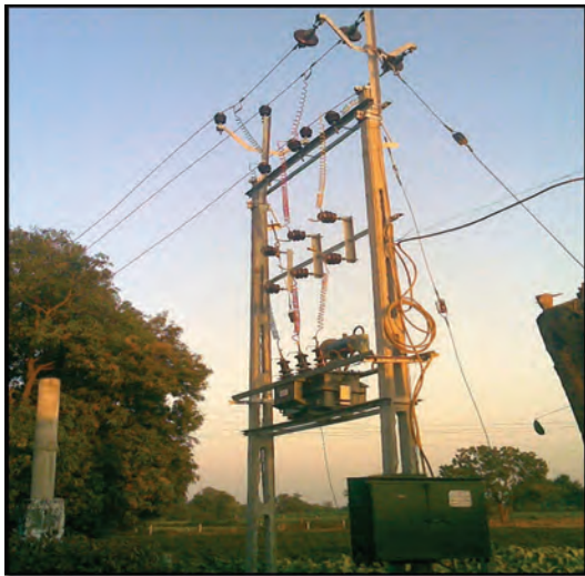
High Voltage Distribution System (HVDS) work at 11 KV Baroda feeder at pilot site Umreth, Gujarat.
