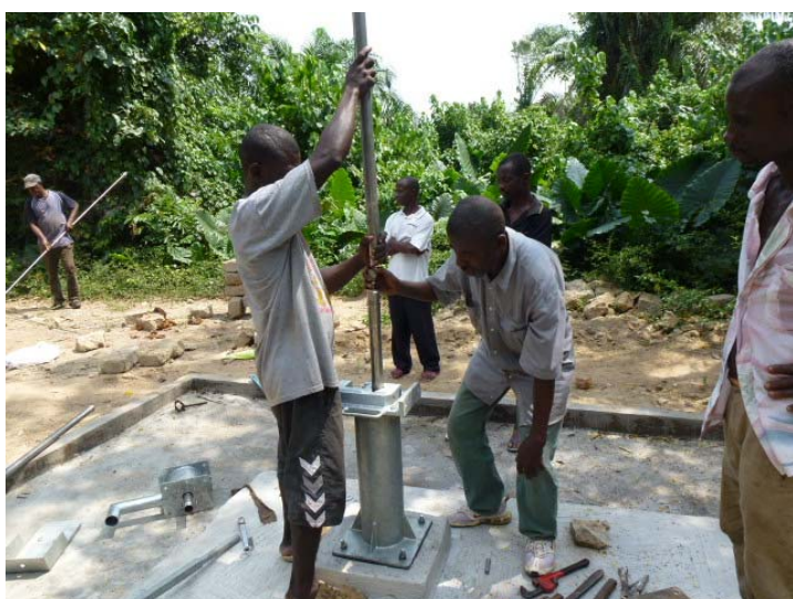
GWASH-trained artisans conduct a major borehole repair on broken-down facility in Nyamebebu in Central Region.
