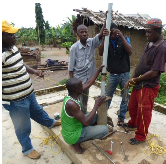
A minor borehole repair on broken-down facility in Kruwa community in Central Region.
