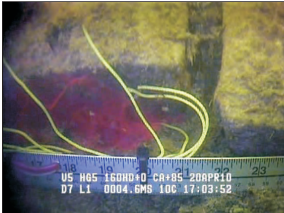
Image 1-1: 2010-04-20-1703 - Joint offset at joint O9 and upper horizontal joint.
