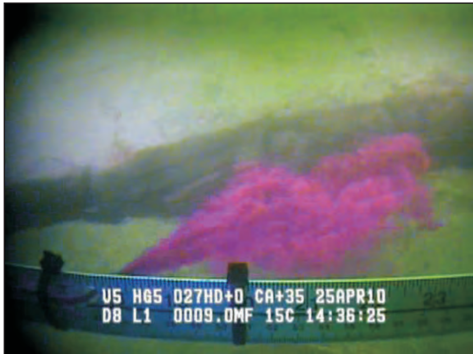
Image 1-16: 2010-04-25-1436 - Dye being pulled in to large leak in joint O1
