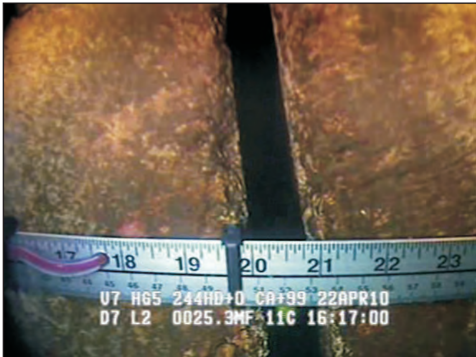
Image 1-6: 2010-04-22-1617 - Large leak closeup at joint 24.
