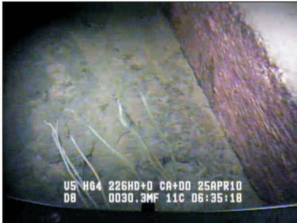
Image 1-11: 2010-04-25-0635 - Raised slab along joint C.
