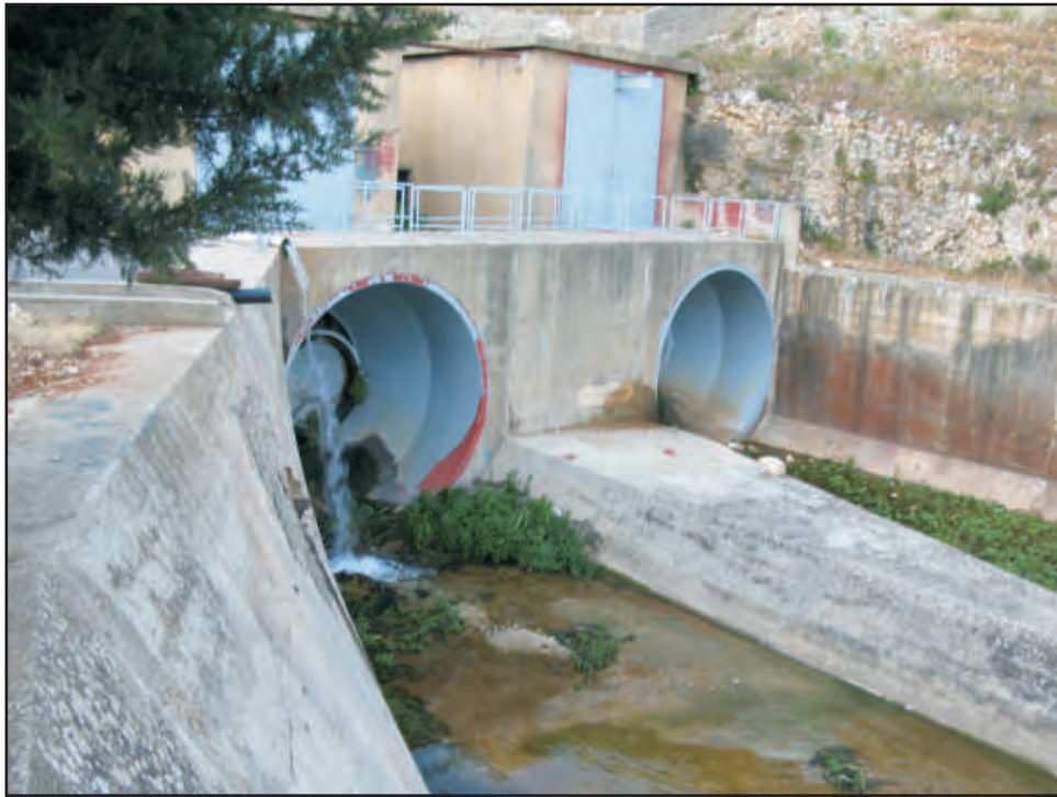
Image 4-7: Drainage outlets with combined leaks in small conduit.
