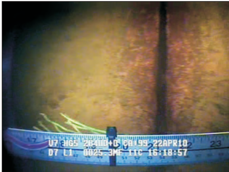
Image 1-7: 2010-04-22-1618 - Large leak in vertical joint 24 at 831.3 m elevation.
