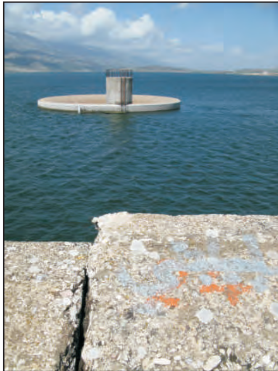
Image 4-4: Spillway and offset at joint 24.
