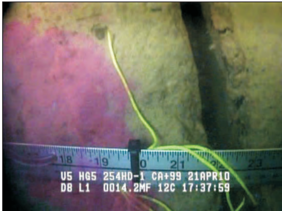
Image 1-4: 2010-04-21-1737 - Leak in vertical joint 29.
