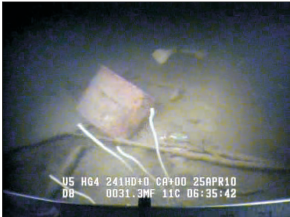
Image 1-10: 2010-04-25-0635 - Debris at bottom of abutment.
