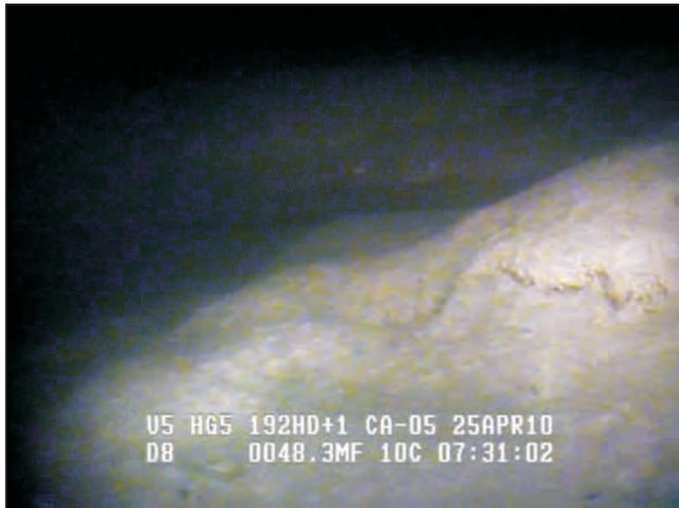
Image 1-12: 2010-04-25-0731 - Silt at floor of power tunnel inlet.
