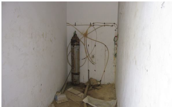
BWE Chlorination Station to be Upgraded
