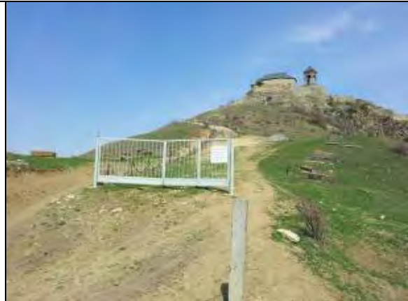
End point of the road to Gorijvari. Land cover shows signs of erosion despite very small 'catchment' of the concrete trail to the Church.
