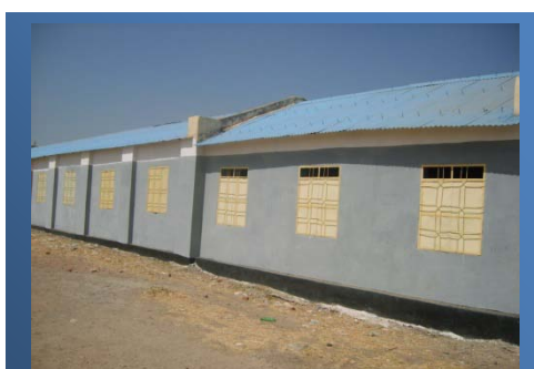
BRIDGE funded renovation of the Bentiu B Girls School in Unity State, which is now providing an enhanced learning environment for 800 students.
