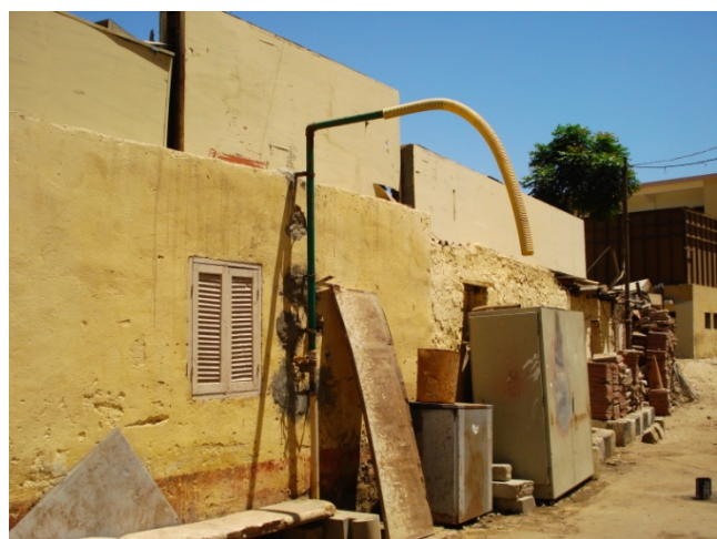
Illegal and Unmetered Connection in Luxor
